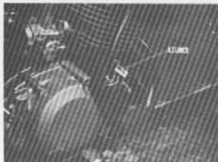
H1 with original H.T. wiring
